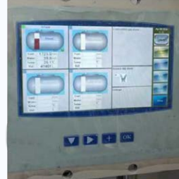
Level gauge system
